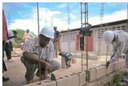
In the two years since the earthquake, MCC engineers trained scores of construction workers and masons in techniques to make buildings safer and more earthquake resistant. As workers such as Guy Evans, left, and Gubeau Jean Ederns lay blocks for three new classrooms at Institution Chretienne de la Grâce, they draw on training and planning by these structural engineers. In addition to funding the current construction, MCC contributed to the first phase of the school's rebuilding by providing a structural engineer to draw the site plan and work alongside masons to build an initial three classrooms.
